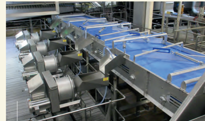
Four Tridis 240P machines integrated in a high capacity French fry production line.
